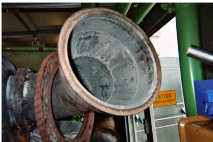
Siloxane deposits in engine exhaust line
