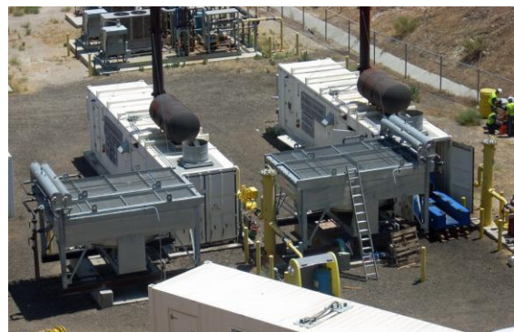
LEG to Electricity Plant "Genset"
